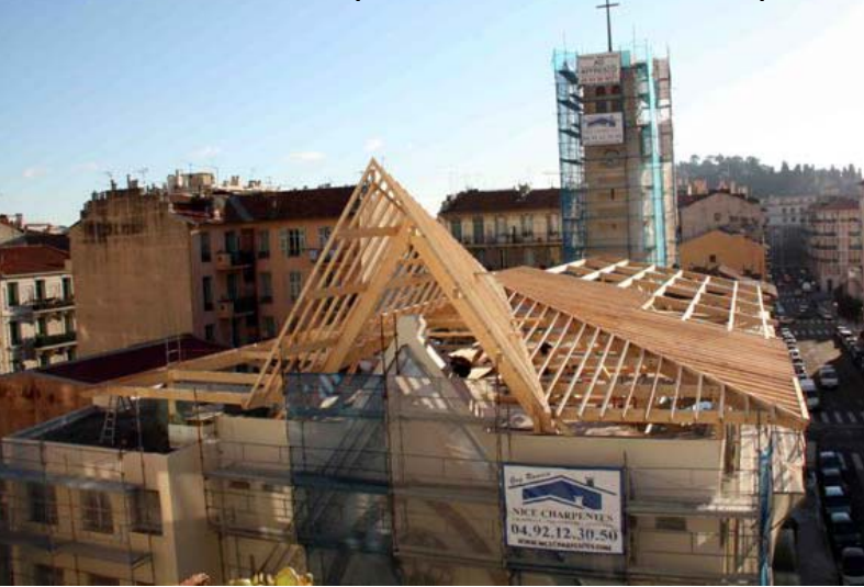
Saint Joseph Church - Structure in spruce and oak for the bell tower - Nice (France)
